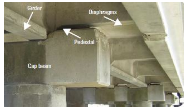
Figure C-32. Girder Design Creating Trapped Air (Chen et al. 2007 with funding from USGS)
