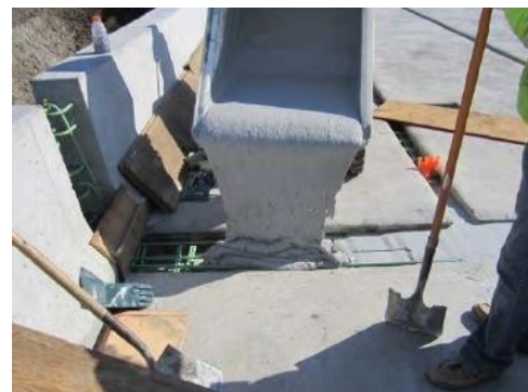
Figure C-103. UHPC Poured into Place (Used with permission © Iowa Department of Transportation, Evans 2017)
