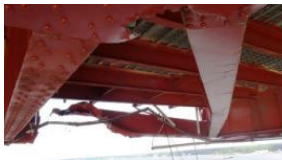
Figure C-54. Severed Tension Chord (Courtesy of Sanya Watts, Watts 2013)
