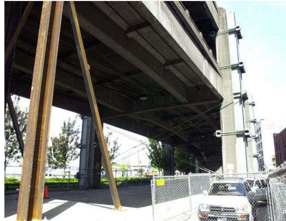
Figure C-11. Temporary Supports After Nisqually Earthquake (Photo by Erik Stuhaug, Courtesy Seattle Municipal Archives (113883))
