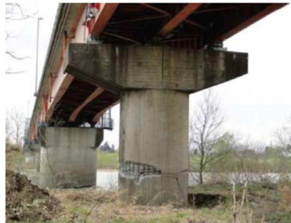
Figure C-4. Fuji Bridge Damage (Kawashima & Matsuzaki, 2012)
