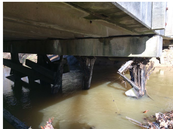
Figure C-18. Debris Damaged Columns (Courtesy of Heavy Bridge Maintenance, ARDOT)
