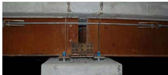
Figure C-104. Post-Tensioning over Pier Cap (Used with permission © Iowa Department of Transportation, Evans 2017)
