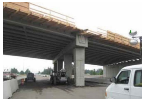
Figure C-123. Architectural Column and Pier Cap Detailing (Courtesy of PCI Journal, Khaleghi et al. 2012)
