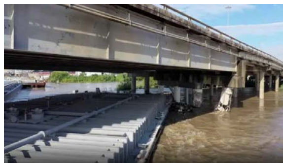
Figure C-62. Severe Column Damage from Barge Impact (Clement 2019)
