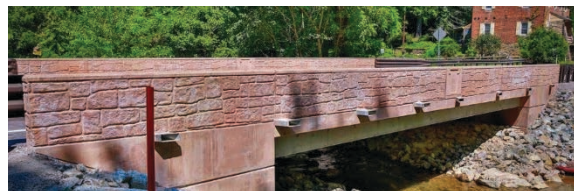
Figure C-75. A Bridge Built part of the P3 Project (Plenary Walsh Keystone Partners 2019)
