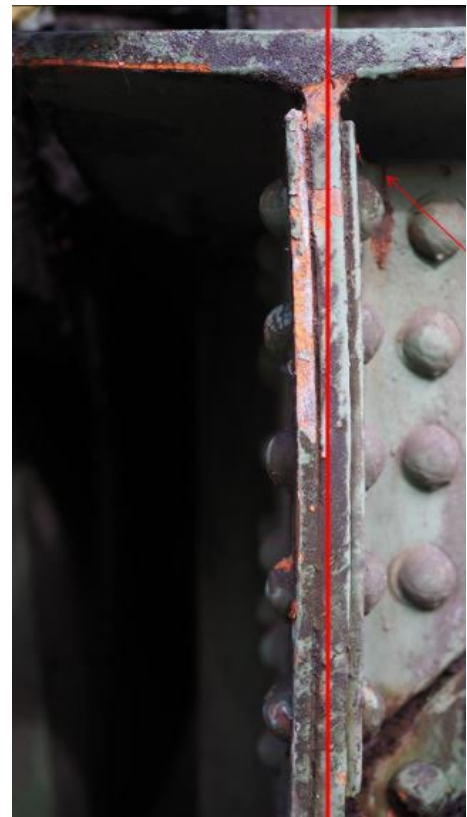
Figure C-69. Floorbeam Buckling (Dobson 2017)
