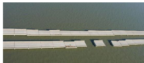
Figure C-28. Aerial View of Damaged and Missing Spans (Alipour 2016)
