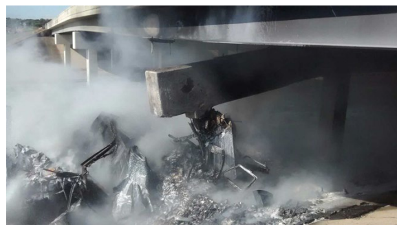
Figure C-48. Damage to Bent (Courtesy of Heavy Bridge Maintenance, ARDOT)
