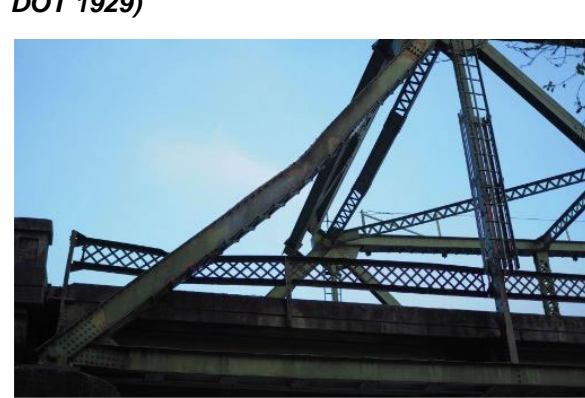
Figure C-67. Side View of Member Distortion (Dobson 2017)
