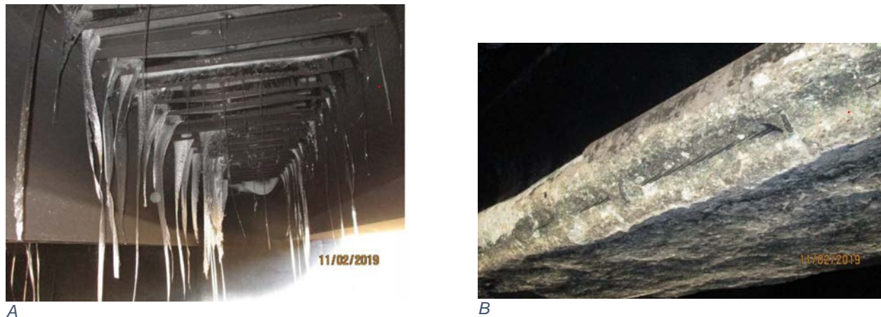
Figure C-38. Fire Damage (Used with permission © Iowa Department of Transportation, HDR 2019) (A) Stay-in-Place Construction Forms and Cross Bracing (B) Spalled Concrete
