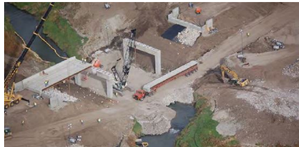
Figure C-99. Aerial View of Construction Site with Culverts (Used with permission © Iowa Department of Transportation, Evans 2017)
