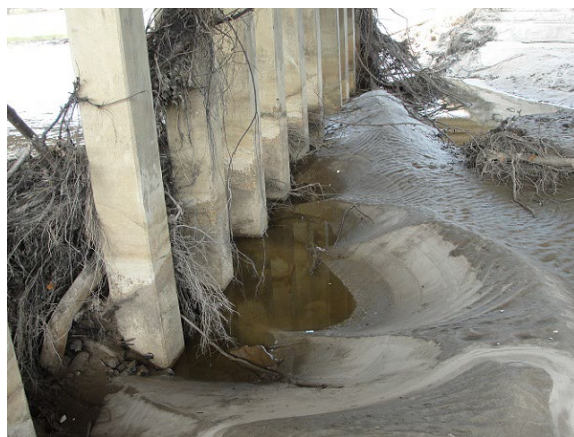
Figure C-23. Scour Damage at Bent (Images courtesy of Padgett et al. 2018)
