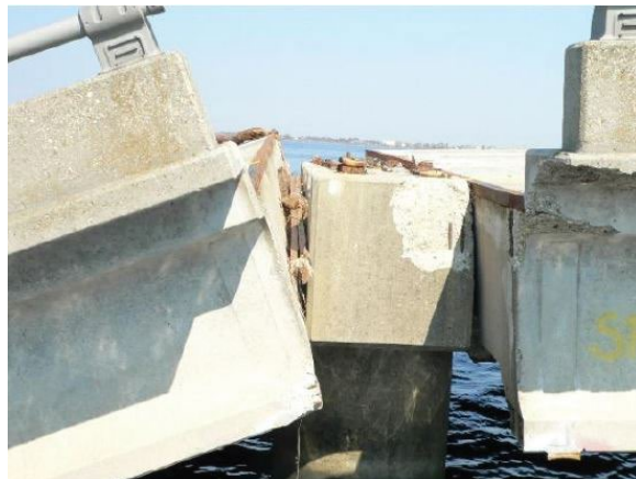
Figure C-31. Girders Fallen off Bent (Alipour 2016)
