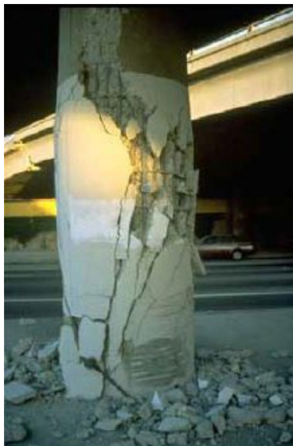
Figure C-16. Typical Column Spalling Damage (Marsh & Stringer 2013)
