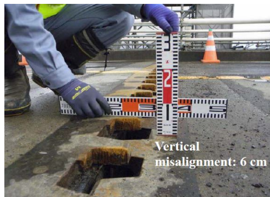
Figure C-3. Earthquake Damage Observed Yuriage Bridge Damage (Japan Bridge Engineering Center 2011)
