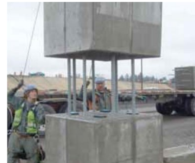
Figure C-121. Setting of a Column Segment (Courtesy of PCI Journal, Khaleghi et al. 2012)
