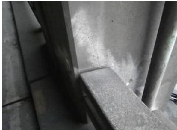
Figure C-9. Cracks from Continued Column Settling (Lindblom 2014)
