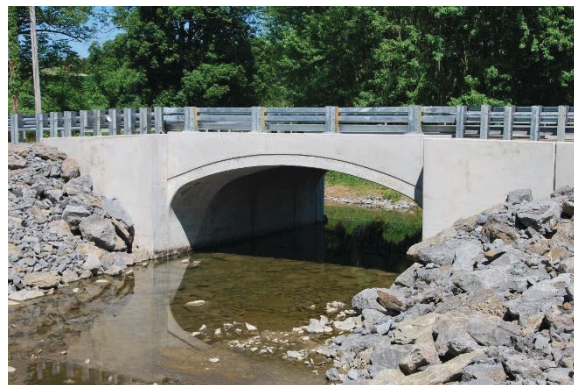
Figure C-76. A Bridge Built part of the P3 Project (Plenary Walsh Keystone Partners 2019)
