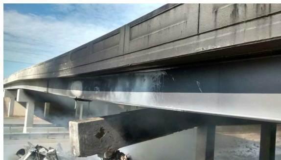
Figure C-49. Damage to Bent (Courtesy of Heavy Bridge Maintenance, ARDOT)
