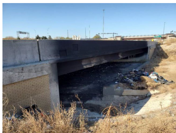
Figure C-36. Fire Damage to I-29NB Perry Creek Conduit Bridge (Used with permission © Iowa Department of Transportation, HDR 2019)
