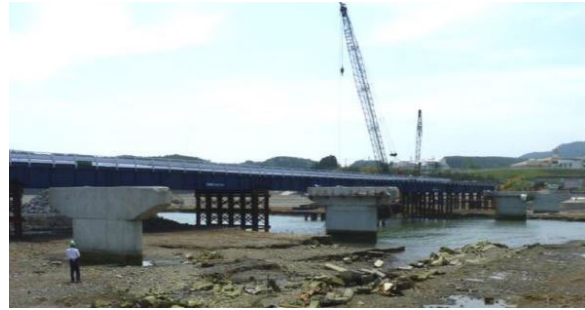
Figure C-5. Koizumi Bridge Damage (Istrati et al. 2017, photo by E.V. Monzon)
