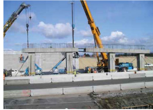
Figure C-122. Setting of a Pier Cap Segment (Courtesy of PCI Journal, Khaleghi et al. 2012)
