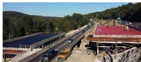
Figure C-96. Aerial View of Construction Site with Nearly Completed Bridges (Bhajandas et al. 2014)
