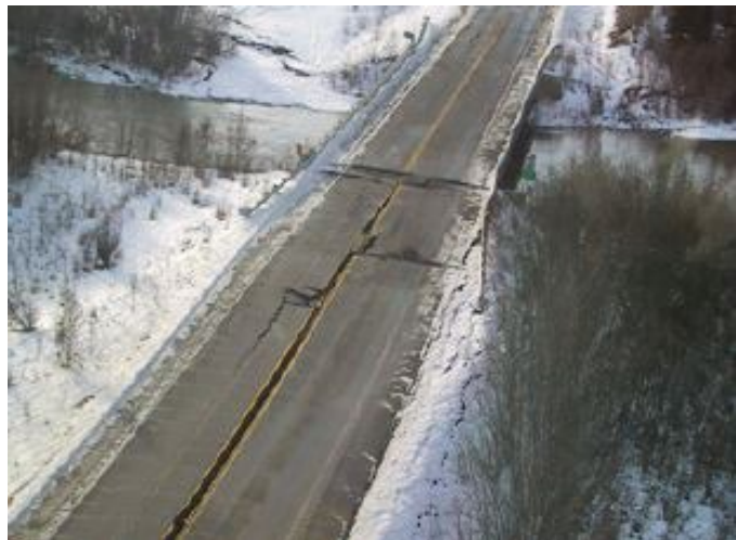
Figure C-1. Shifting of the Tok Cutoff Bridge (McCarthy 2003)
